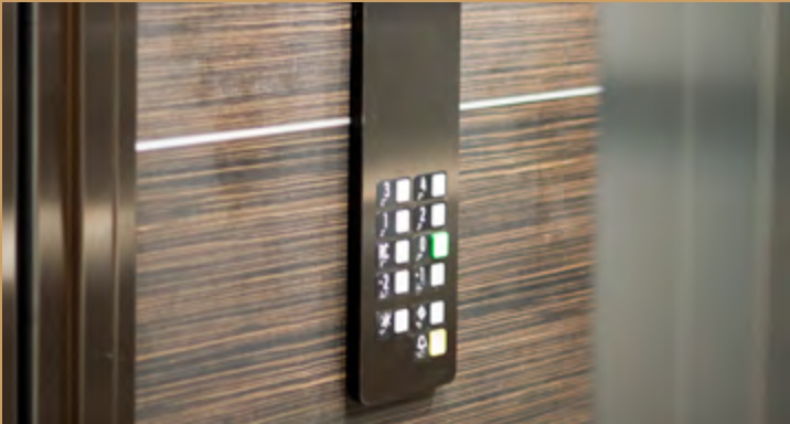
Easy access from your garage to your home Your block is equipped with a lift serving all floors.
